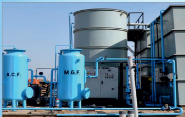
SEWAGE TREATMENT PLANTS
