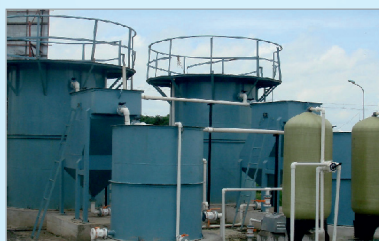
EFFLUENT TREATMENT PLANTS
